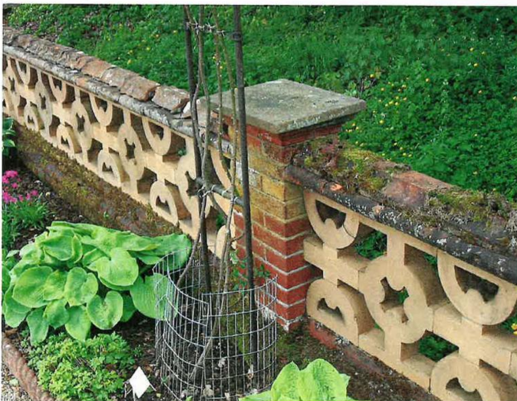
Fig. 26 Ha-ha wall - showing coping damage.
