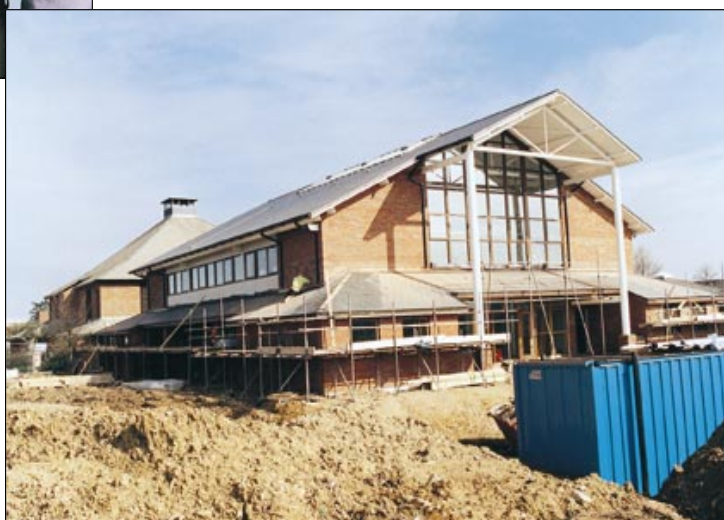
An extension to the Fowden Conference Hall, costing £1.2 million, was started in mid-August 1998 and is scheduled for completion in mid-Summer 1999. The new building will be named after Professor Trevor Lewis CBE, Director of IACR and of Rothamsted 1989-93. This major new facility will enable Rothamsted to host more international scientific conferences and will also provide an important local and regional venue for commercial seminars, training courses and trade exhibitions
