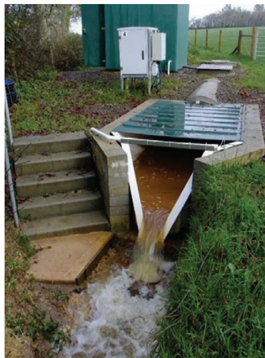
Catchment flumes and instrumentation cabin
